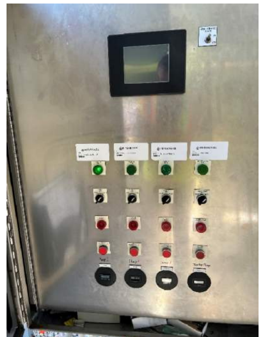
Booster Pump Control Panel 2
