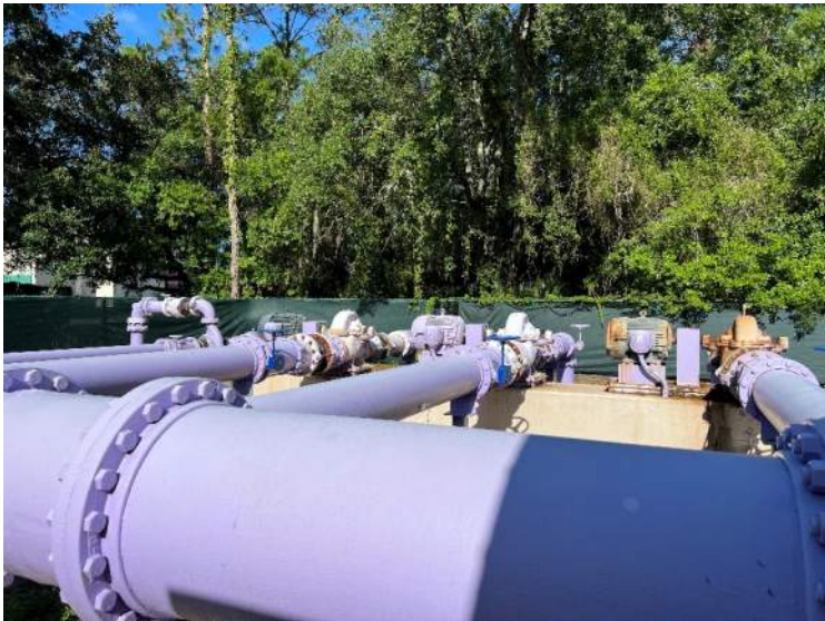
Reclaimed Water Pumps
