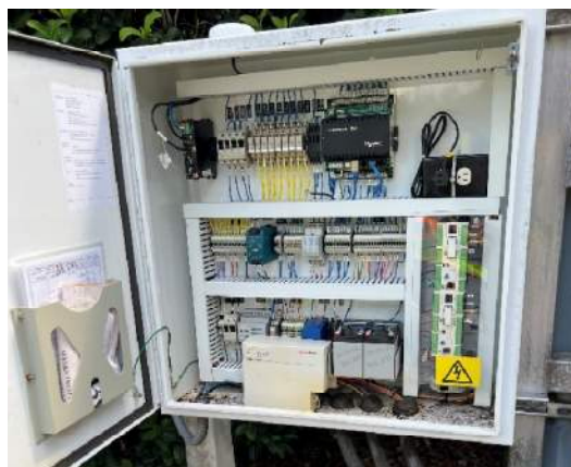
SCADA Control Panel
