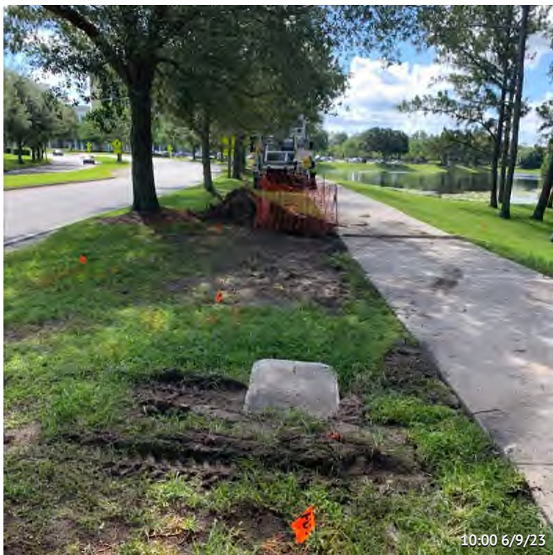
Item 27 More damage
