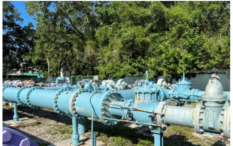
Potable Water Booster Pumps
