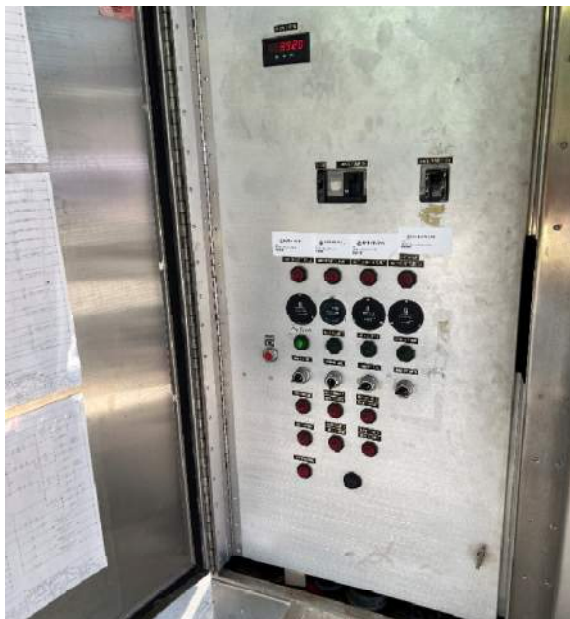
Booster Pump Control Panel 1
